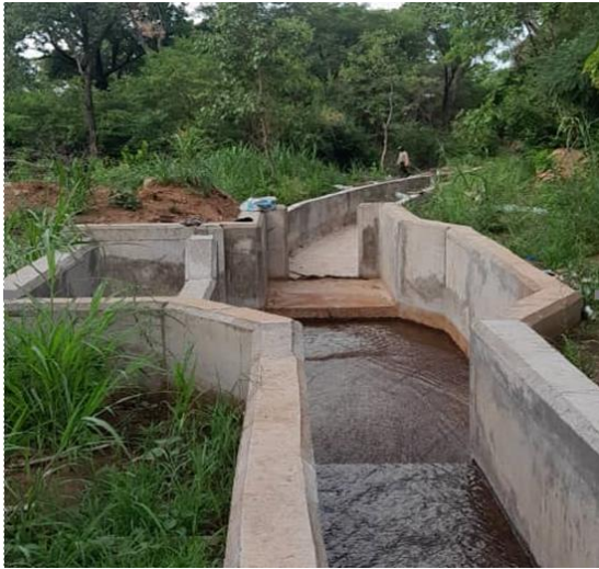
Plate 7: Water control gate at Itamboleo village, Mbarali DC.
