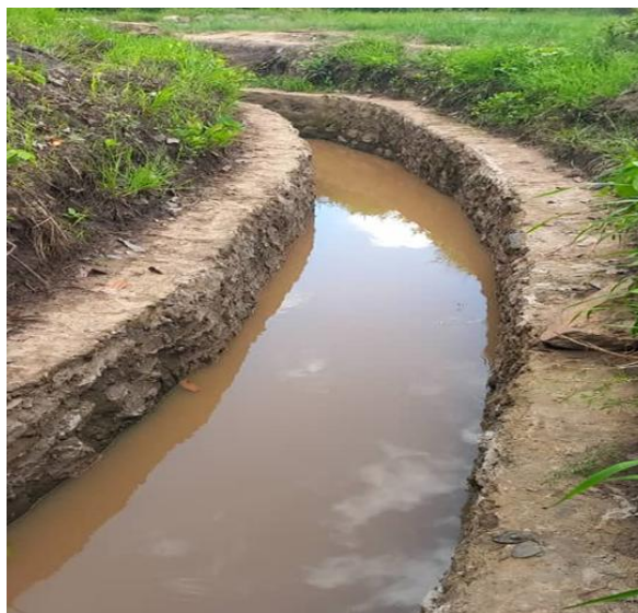
Plate 23: Irrigation canal at the Mnyagala Irrigation Scheme in Nyagala village, Tanganyika DC
